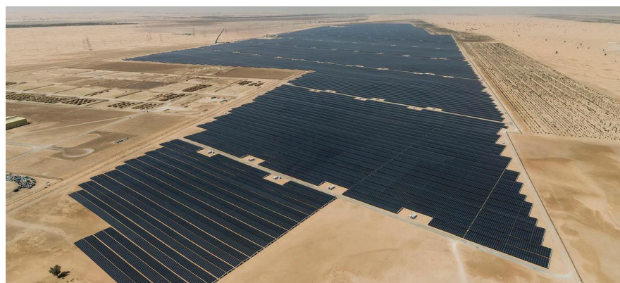
Noor Abu Dhabi, the world's largest solar IPP, uses ENEXSA's settlement system (picture courtesy of Sweihan PV Power Company)
